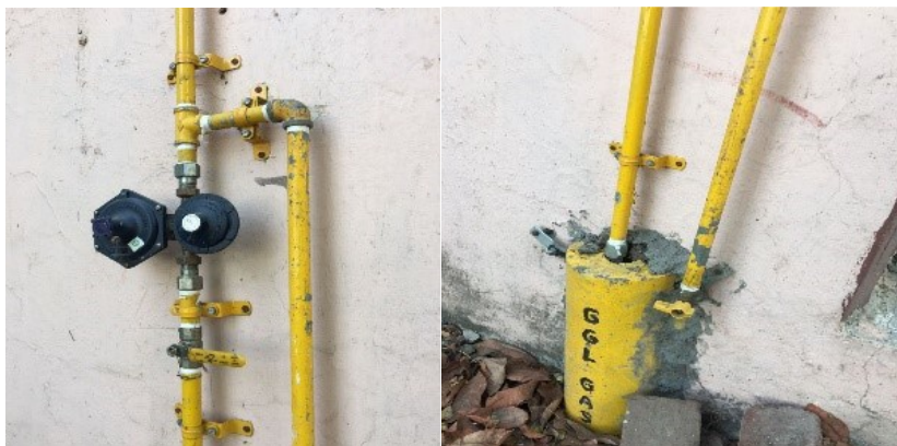
Figure-11: Stagnant riser pipelines and tapping points
